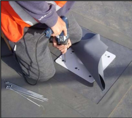
The IFP is positioned and secured in position with appropriate type and length fixings
